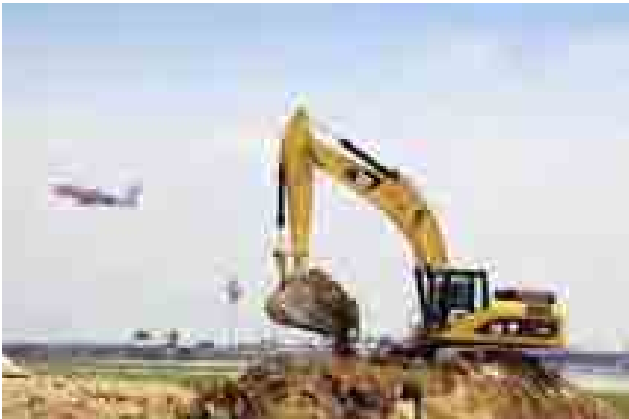
Sime Darby Industrial provided more than 100 units of various Caterpillar machines for the KLIA2 earthworks project
