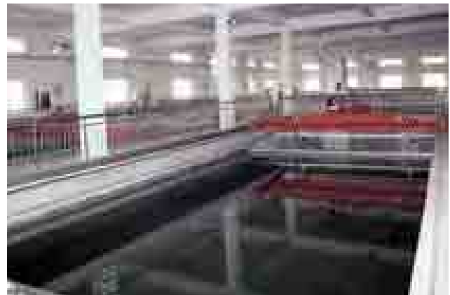
Weifang Sime Darby Water Co Ltd increases its total capacity to 140,000 m 3 per day
