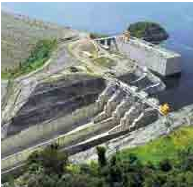
Water elevation work at the Bakun Hydroelectric Dam Project has reached 205.4m as of 15 July 2011
